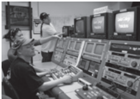
Television Control Room
